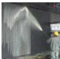
Top photo: Applying and spreading retarder on the bottom of formwork. The retarder is applied with a broom and spread with a paint roller.
