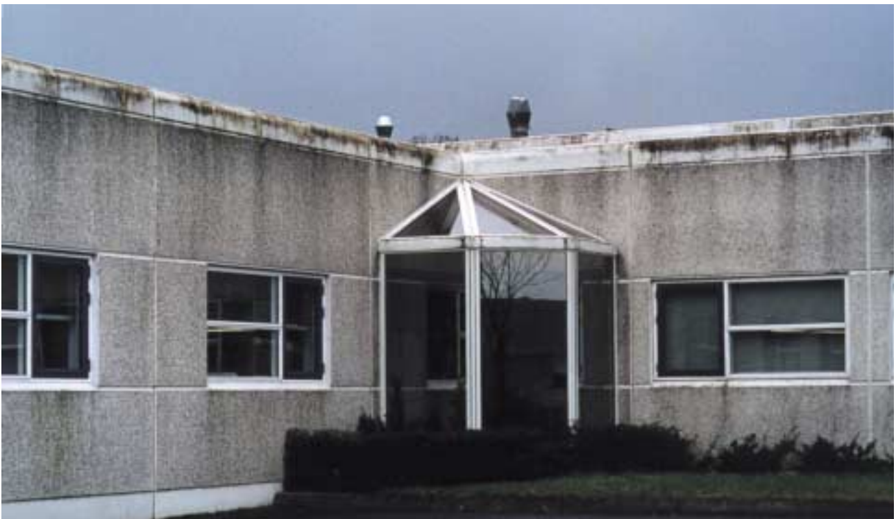
Strong discoloration can be avoided by rainwater being appropriately drained off.
