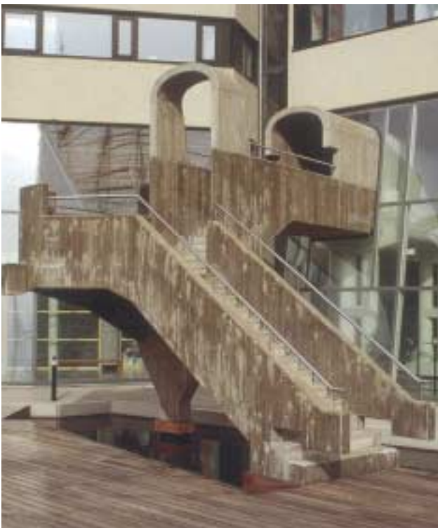
Coloured concrete with coloured efflorescence.
