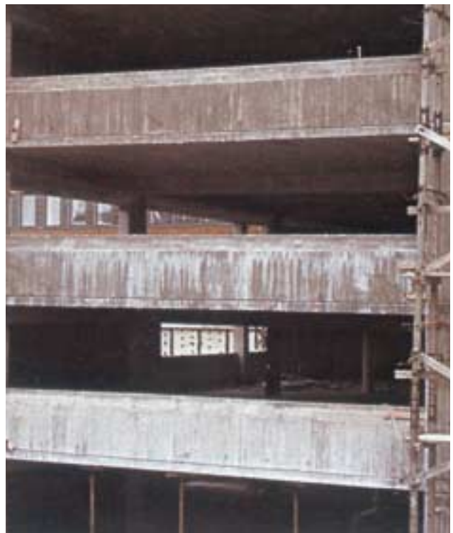
Efflorescence caused by casting during the cold and rainy time of the year.
